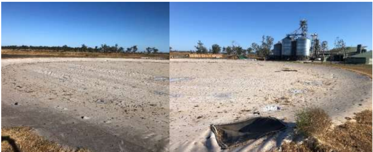
Figure 24: EvapCap continuous floating cover installed at Wainui Feedlot showing maintenance repair in the bottom right (Photo: Matt Siebur)
