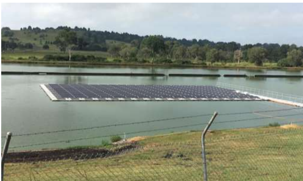
Figure 13: Floating photovoltaic panels installed at the East Lismore Sewage Treatment plant
